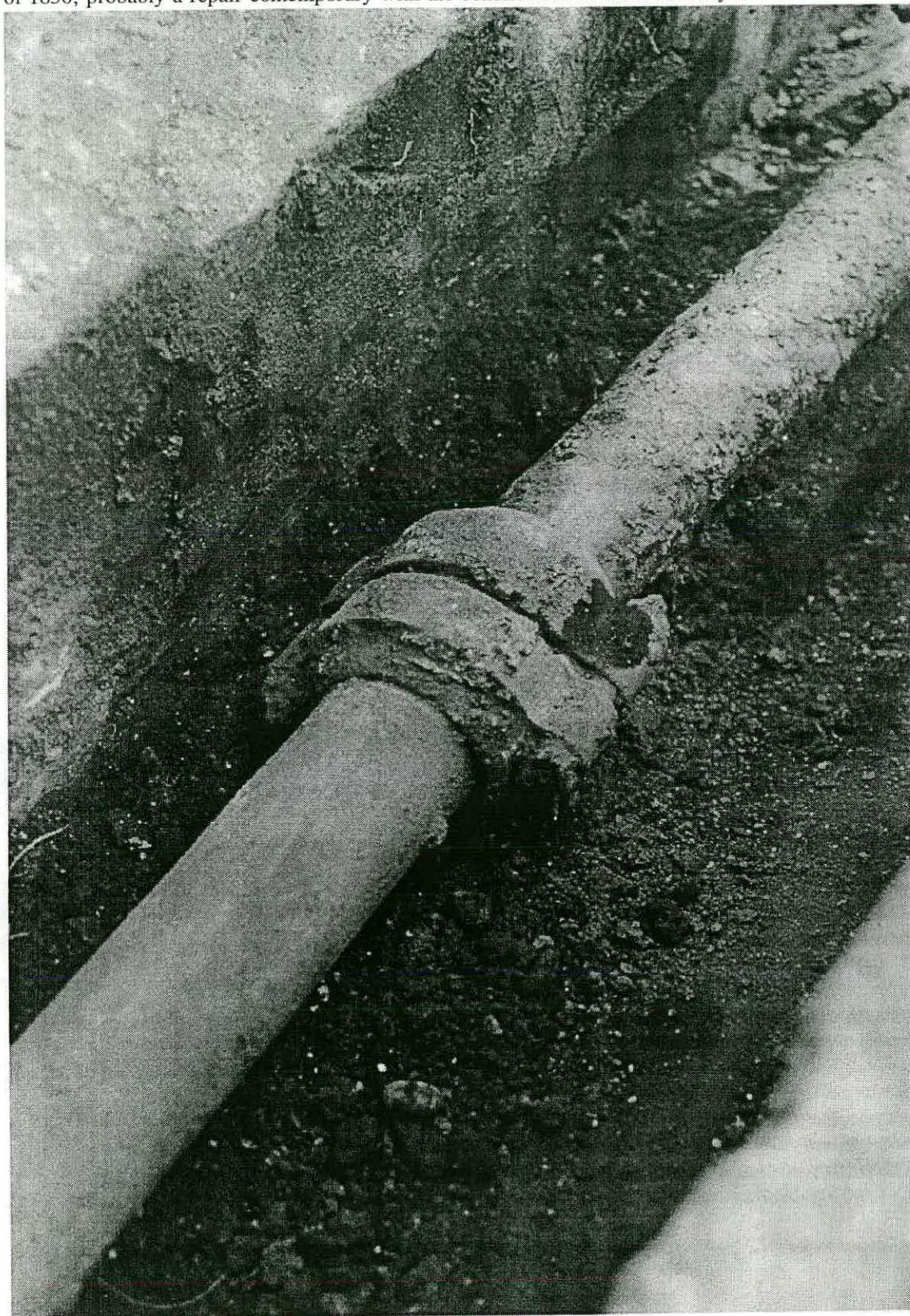
Figure 20 A bolted joint in the 2" pipes in the channel on the north side of the first greenhouse of 1856, probably a repair contemporary with the construction of the laboratory in 1881
